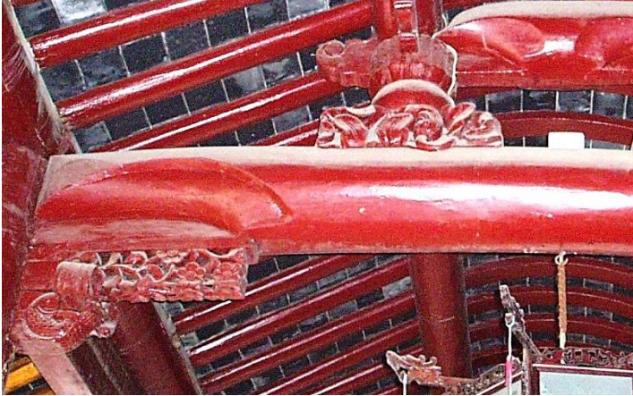
Fig.263. Detail of the carvings of the eave structure of the prayer hall, Xianhe Mosque, Yangzhou.
