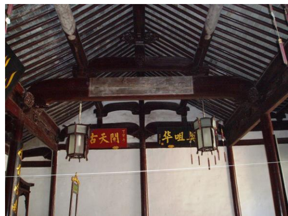
Fig.49. Detail of the structural frame of the prayer hall, Songjiang Mosque, Songjiang.
