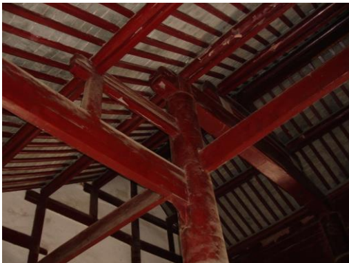
Fig.61. Detail of the structural frame of the prayer hall, Luhe Nanmen Mosque, Nanjing.
