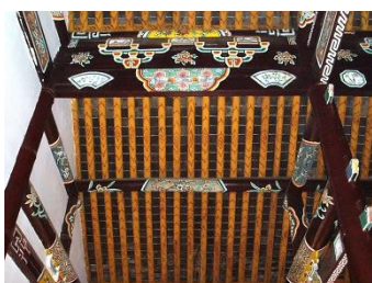
Fig.272. Detail of the beam paintings in the prayer hall, Shanxiang Mosque, Zhenjiang.
