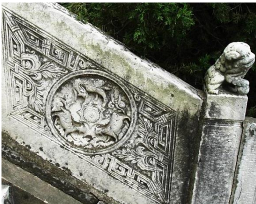
Fig.232. Detail of the decoration on the balustrade, Baha al-Din tomb complex, Yangzhou.
