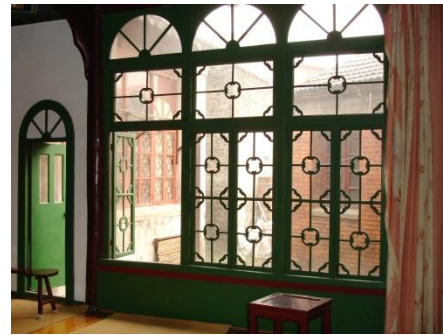
Fig 256. Decorative design of the window screen of the prayer hall, Shanxiang Mosque, Zhenjiang.
