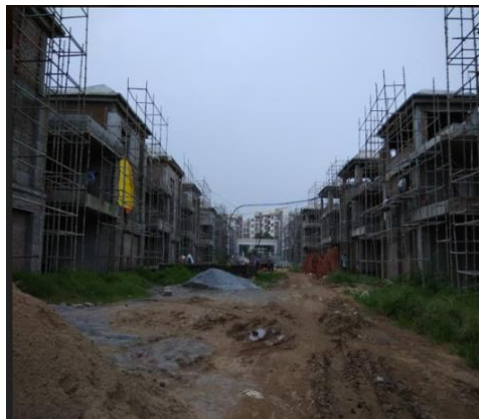
Figure 6.1: Construction Site A – Rishabh Builders and Developers (Source: Photographed by the author, 2019)
