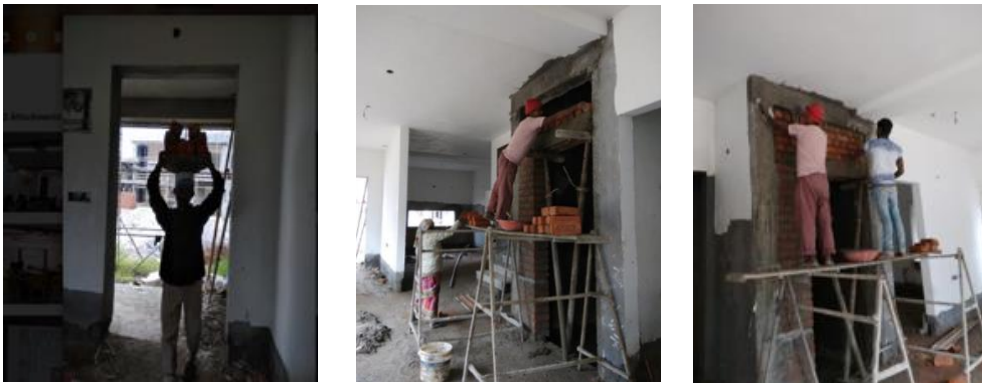
Figure 6.3: A helper transporting bricks (left); and Brick laying and plastering by mistris (centre and right) (Source: Photographed by the author, 2019)
