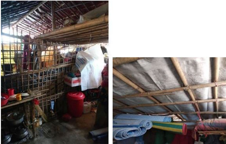
Fig. 6 Left: Use of additional bamboo to create a loft. If these members had been placed at 90 degrees and tied to the wall plates or posts, they would have also formed cross beams. Right: Rafter and purlins made of muli, with purlins placed under the rafters rather than on top
