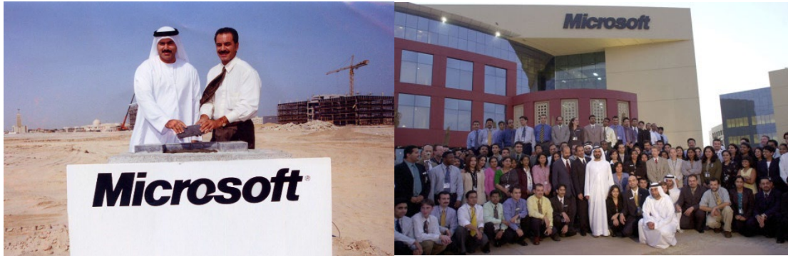
Figure 8.1 HE Mohammad Al Gergawi and Microsoft's Regional CEO laying the foundation stone, Source: Gulf News Archives
