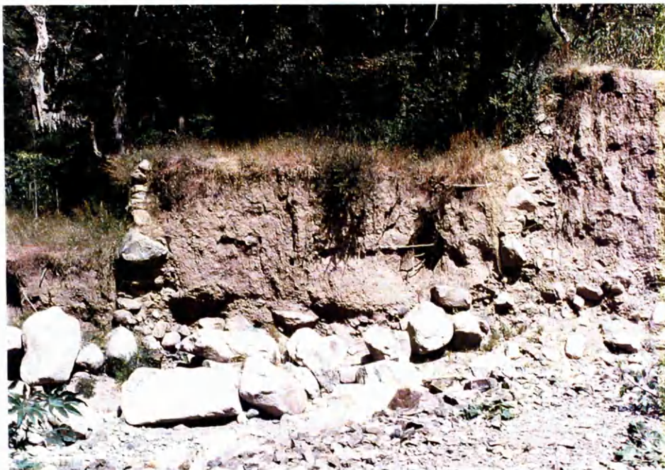
Photo 4: Wadi Terrace Erosion. Wadi Nibaq. Wadi flow has eroded the terraces revealing the intervening walls between three terrace levels.
