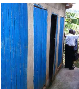
Cramped water closets
