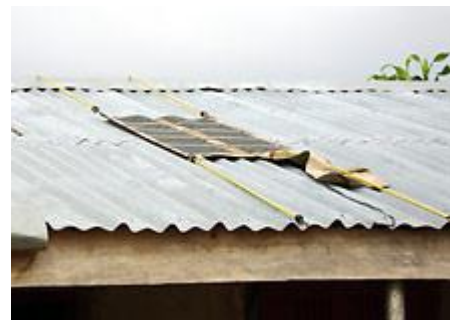
Figure 2 Solar panel on roof
