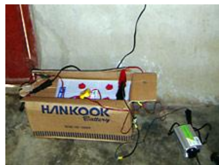
Figure 3 Battery and inverter
